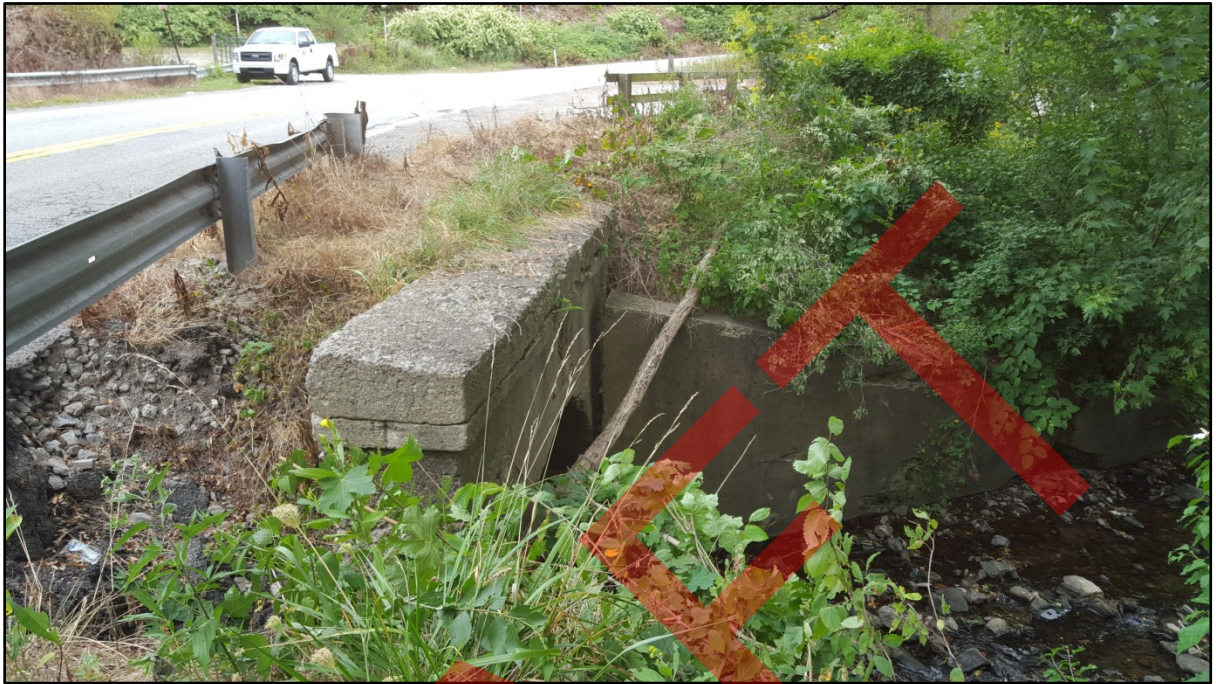
Figure 4-10: Flooding Location at Commercial Street Culvert along Nine Mile Run
