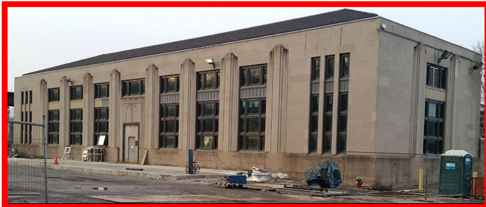
Bruecken Pump Station
