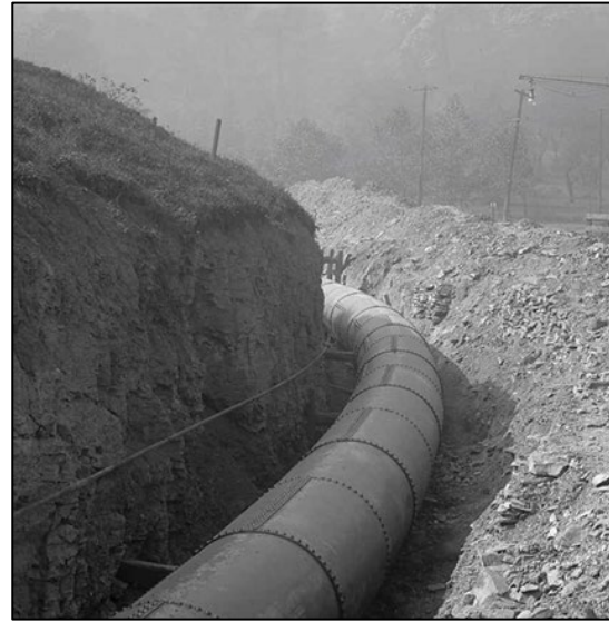
Redundant Lanpher Rising Main
