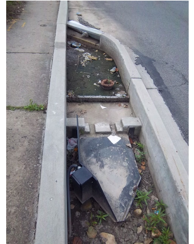
Repeated vehicle strikes damaged trees and infrastructure
