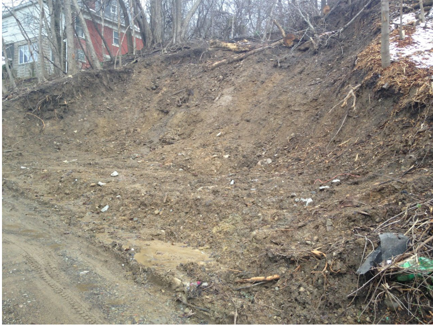
2018 Landslide on Haverhill St.
