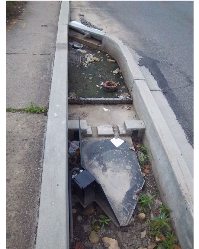
Repeated vehicle strikes damaged trees and infrastructure
