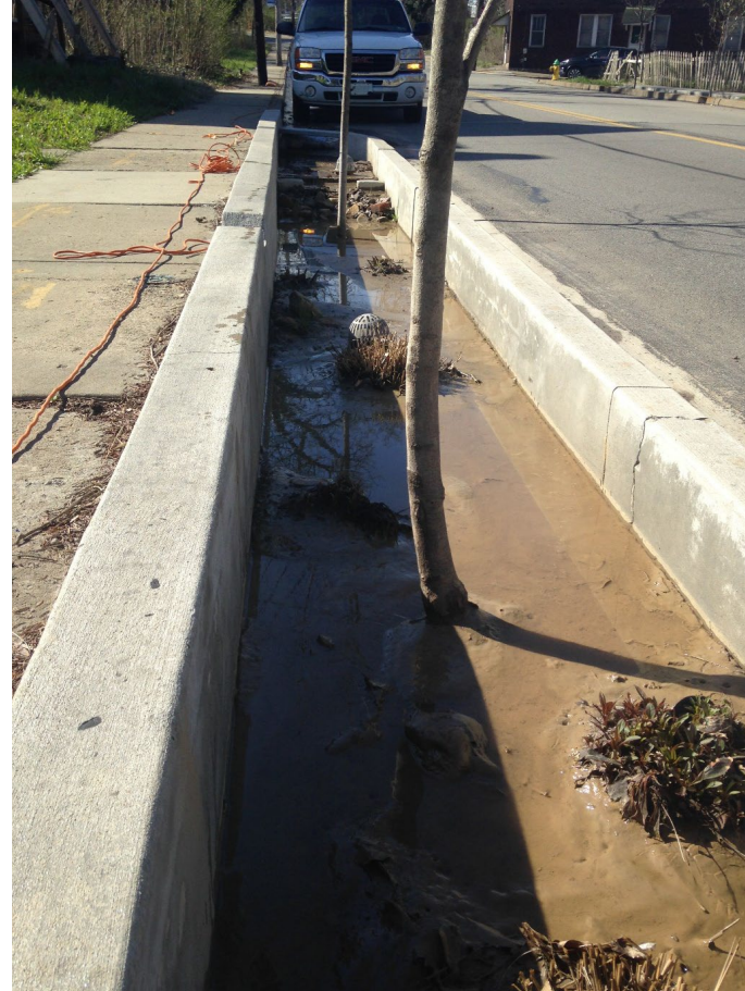
Sediment and seep water inundated stormwater planters
