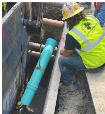
Contractor crews installing the new sewer main on Fuchsia Way in Homewood
