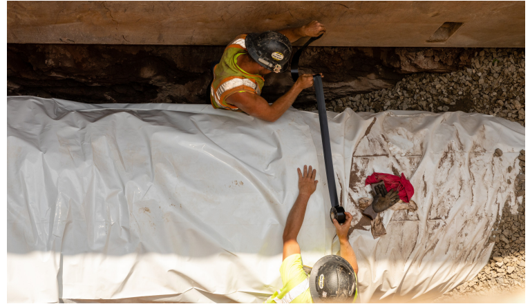
Your ratepayer dollars in action: Aerial view of crews installing a 48" water main in Highland Park. The pipe is wrapped in a protective plastic covering to prevent corrosion from the soil.
