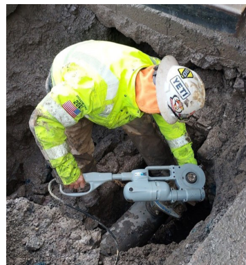
Contractors in the East End begin the replacement of lead lines as part of the Urgent Lead Service Line Replacement Program.
