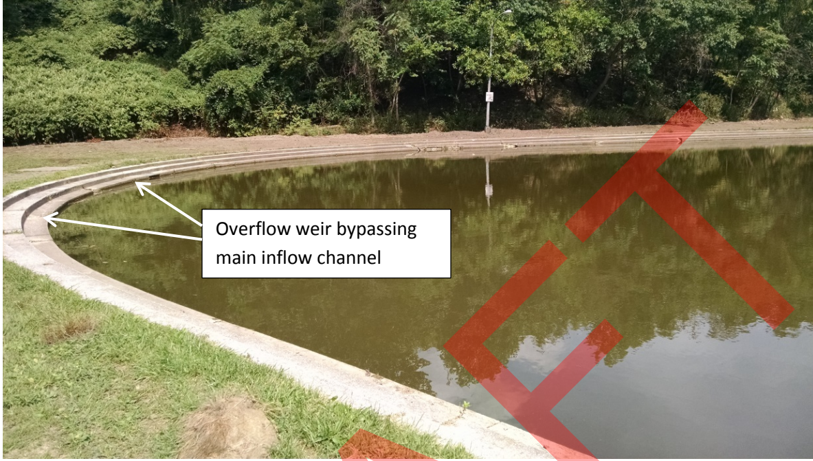
Figure 5-15: Panther Hollow Lake Overflow Weirs Diverting Water to the Lake Overflow Pipe
