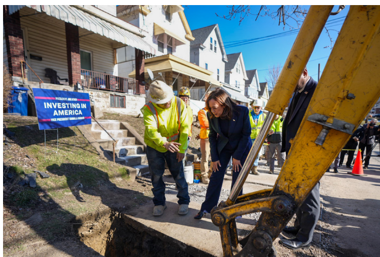
Vice President Kamala Harris visits a PWSA job site where contractor crews removed lead service lines in Pittsburgh's West End.
